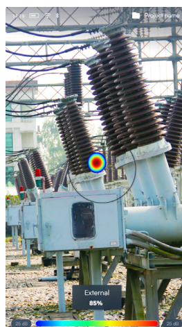
Partial Discharge Detection
