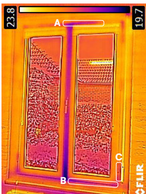
Image 3 - labeled thermal camera airtightness leak visualization
