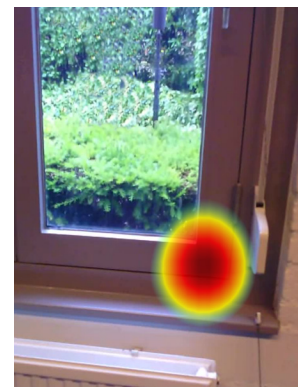
Image 6 - acoustic visualization of leak C
